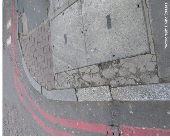
Poor quality pavement Photograph: Living Streets
